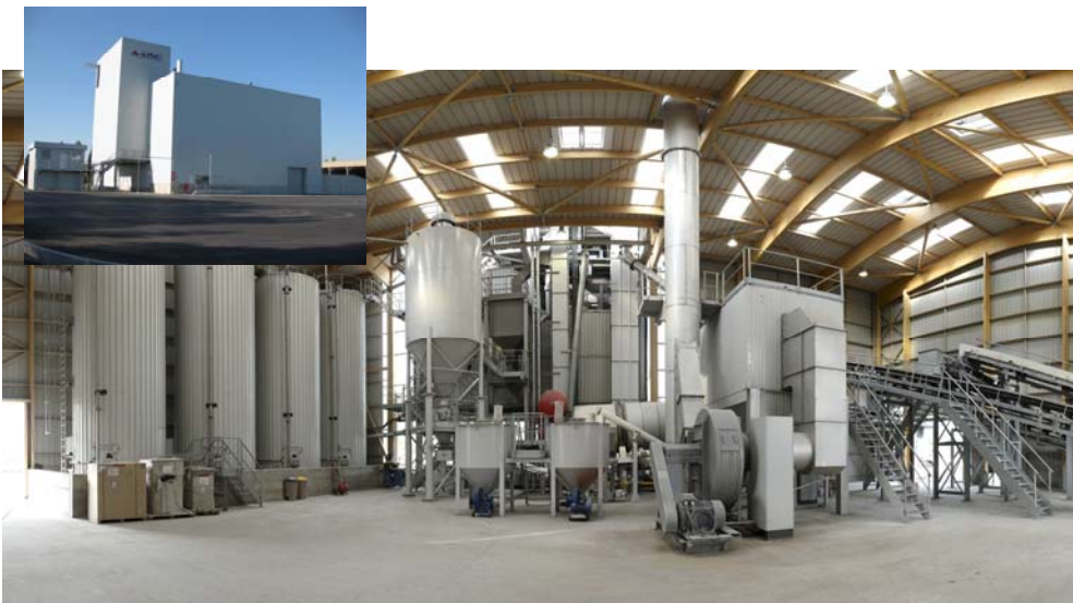
Figure 12: Completely cladded ContiMix plant using compensator technology
