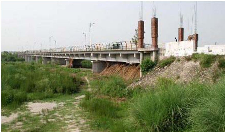
Photo 4 – A view of Bridge constructed over Nasrala Choe village Mankoo on village Road linking Kathar to Fughlana by Sant Baba Bhag Singh Charitable Trust
