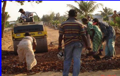
Placement of crushed Tsunami debris as sub-base by labour with hand tools
