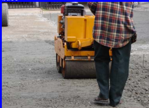
Use of 1Tonne roller for base course compaction; note use of strings and pegs for layer control
