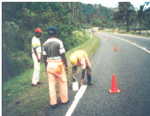
Plate 1 (left): Road marking to improve safety.
