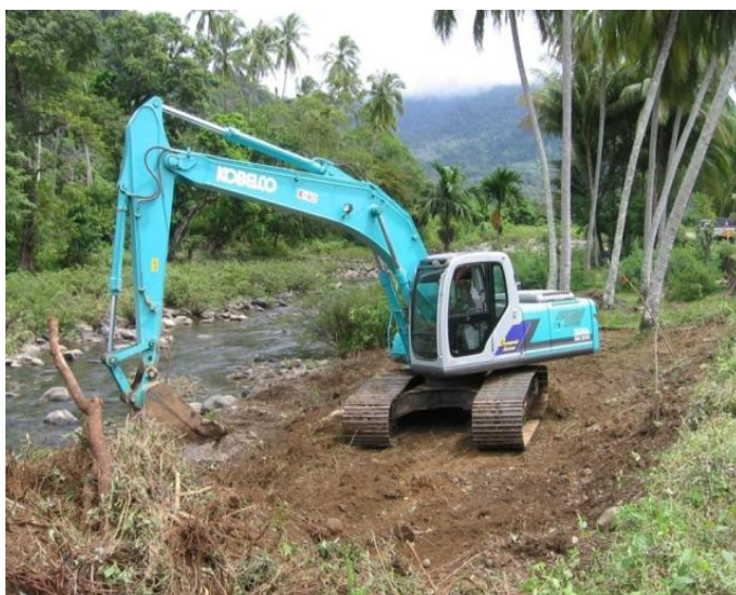
Construction began adjacent to a river in the Aceh jungle in October 2006.
