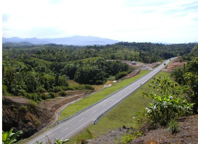
To prevent erosion, topsoil and sod have been installed on all embankment slopes.
