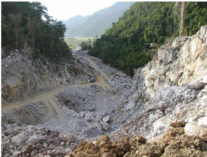
To avoid running along the sandy shoreline, the corridor of the new Aceh Road was blasted through the low point between adjacent limestone and granite hills. A photo of the finished 65m high cut is included in the Summary / Conclusion.
