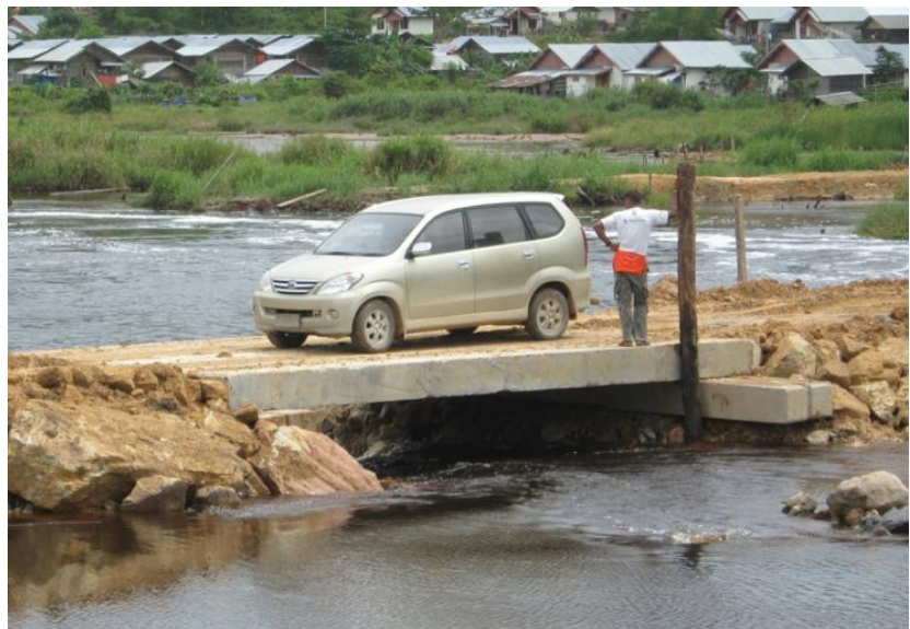
Lageun, Pante Klyon: With the same efficiency and professionalism it demonstrated in April, USAID contractor PT Ssangyong one again responded quickly when it heard the newly erected Bailey bridge had been severely damaged by heavy rains. A temporary crossing was established and made available to the public within 48 hours.
