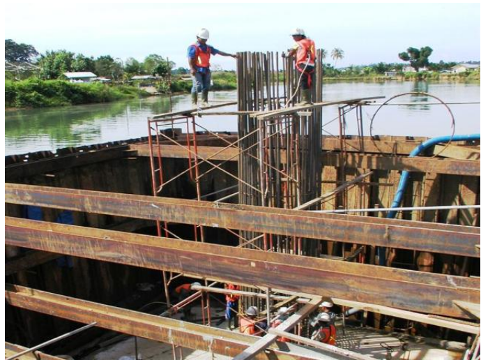
The transfer of technology, knowledge and experience in road construction to the Aceh workforce is contributing to the long term growth of the region.
