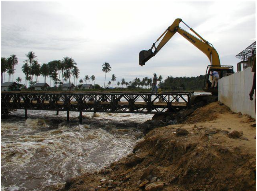
Lageun, Pante Klyon: Using large boulders as reinforcement, USAID contractor PT Ssangyong prevented a newly erected Bailey bridge from being washed away after surging waters had burst through the dirt road that served as the bridge's southern abutment.
