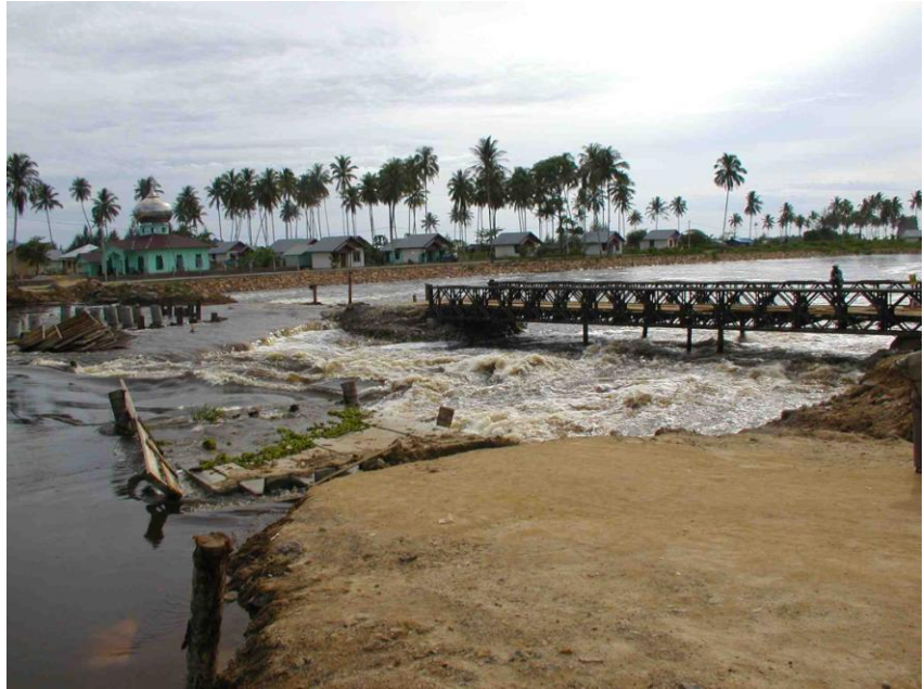
Lageun, Pante Klyon: Although Aceh's monsoon season usually ends in February or March, May 2009 saw five successive days of heavy rain caused severe flooding across much of Aceh. The force of the water rushing down rivers broke through levee banks, destroyed estuary and harbor embankments, and swept away bridges. Some 18 kms north of Calang, a sand embankment supporting a newly erected Bailey bridge was washed away, almost taking the bridge with it.
