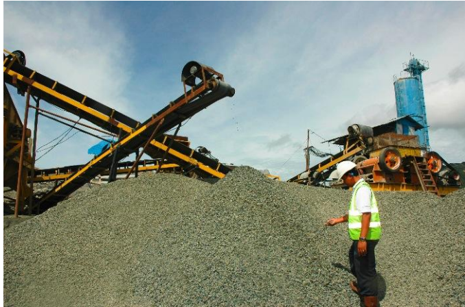
A quality control engineer inspects the quality of gravel used to make the embankment and concrete.
