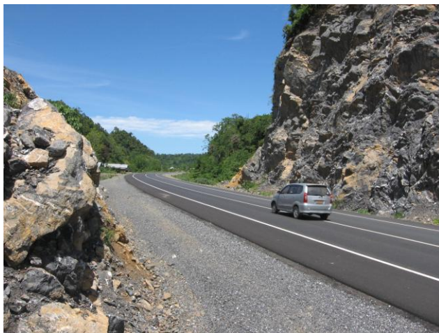
Providing a more direct and safer alignment required blasting through limestone hills.
