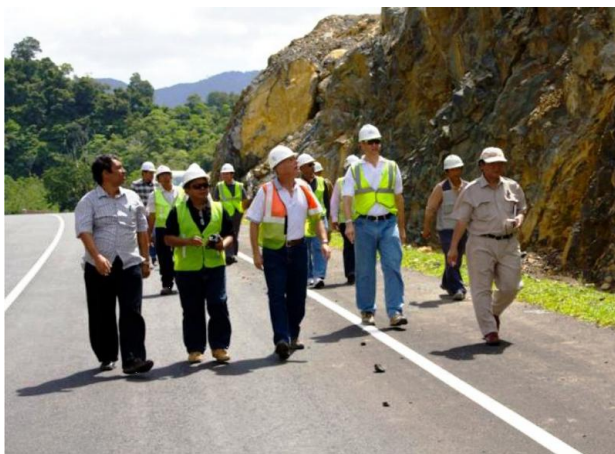
Site walk with representatives of USAID, the Indonesian Government, the construction management contractor and the construction contractor to inspect a completed segment for deficiencies prior to the start of the one-year warranty period.
