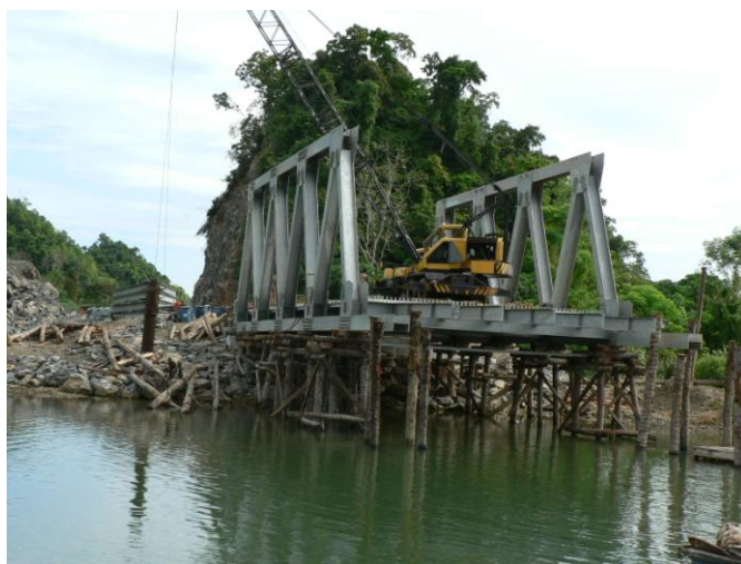
In accordance with local standards, rudimentary construction methods were frequently employed, such as the use of coconut palm scaffolding to support the erection of steel bridges.
