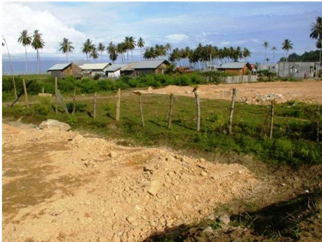
Construction often had to be suspended while access was obtained to the Aceh Road corridor including at this 50m stretch.
