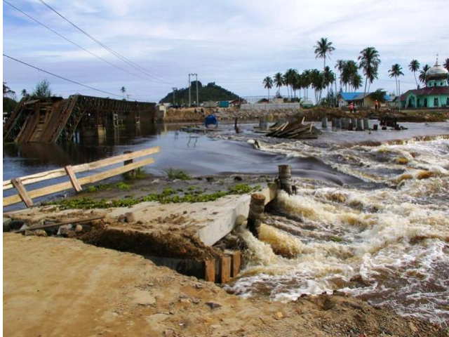
A surge in a river following days of heavy rain washed away a temporary river crossing at the site of the construction of a new steel truss bridge. A collapsed Bailey bridge can be seen on the left as can piles for the new bridge's center pier foundation on the right.
