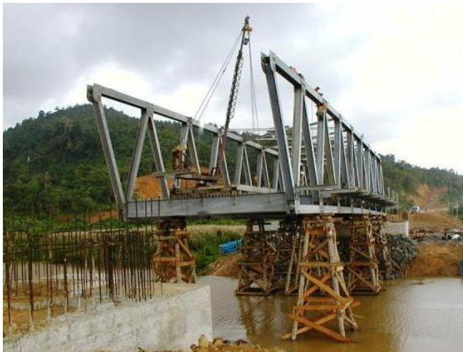
Local construction methods were frequently employed, such as the use of coconut palm towers to support the erection of steel bridges.
