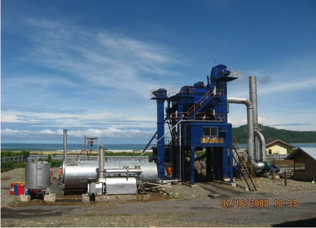
The asphalt mixing plant at base-camp I Jantang village, Aceh, produces asphalt for the section of road being built by the prime contractor, PT Hutama Karya.
