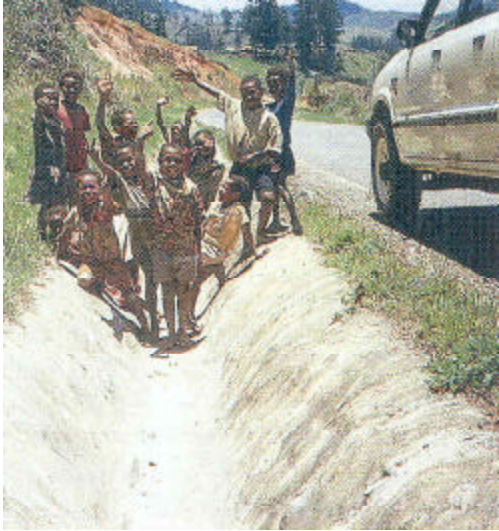
Plate 3: Potentially dangerous deep V-type ditches in Papua New Guinea.
