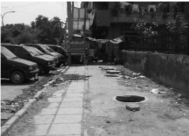
Patparganj: Potholes endanger pedestrians close to Ramkrishna Apartment
