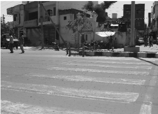
Patparganj: Zebra crossing hits high curb heights
